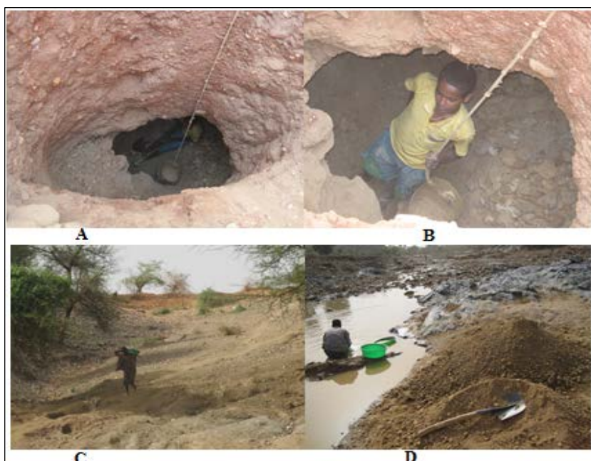
Fig.3: Partial view of small scale gold mining, dangerous working condition (e.g. pit without support), in Asgede Tsimbla.
